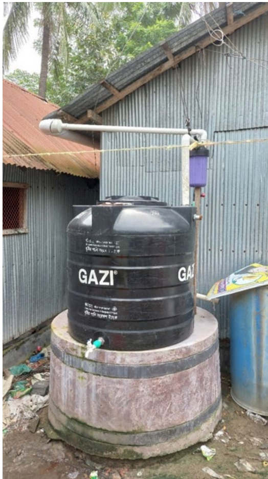
Figure 11: Rainwater harvesting plant
