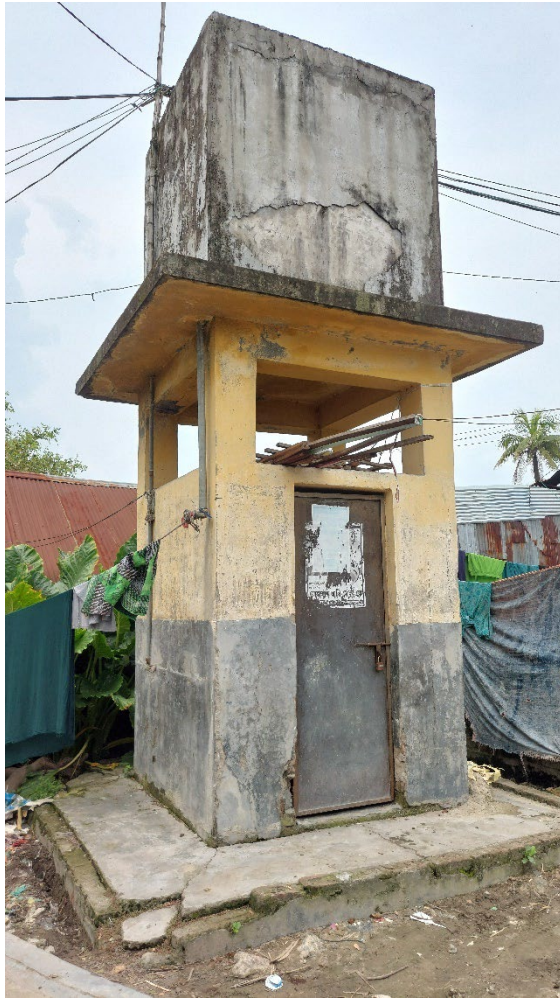
Figure 13: A nonfunctional old water supply tank
