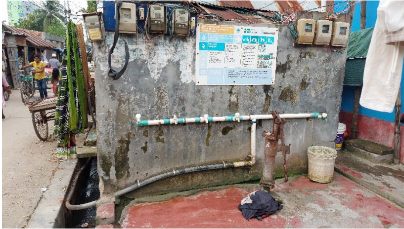
Figure 19: Water supply pipeline from the submersible pump outside Nurani Mahalla
