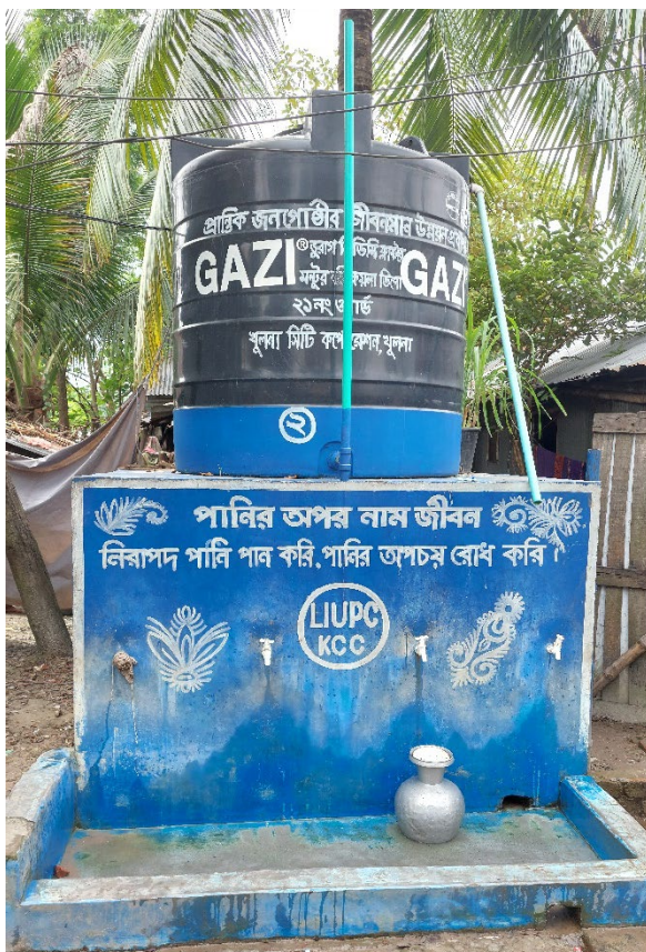
Figure 10: Submersible pumps for drinking water supply
